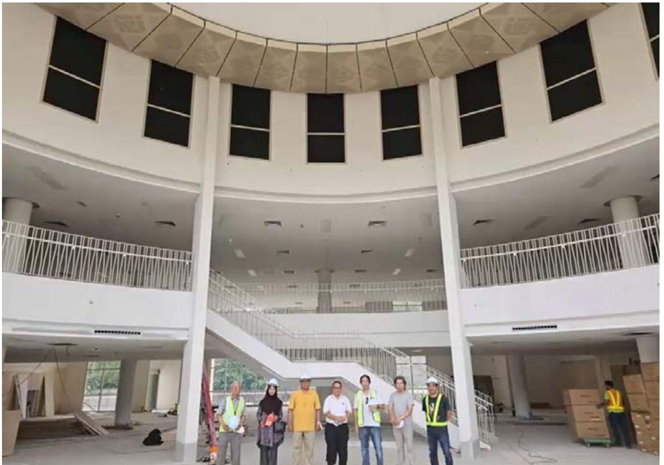
Members of the BTF making a site visit on 13th January 2024 at the main lobby. (Left to Right) Mr Choo Choon Yeow (MAGI Project Manager), Dr Norsiah Ali, Dato' Paduka Dr JP Kamalanathan, Associate Professor Dato' Dr Mohammad Husni, Tan Sri Datuk Dr Ridzwan Bakar & Mr Azan Azril (GDP Architects)
